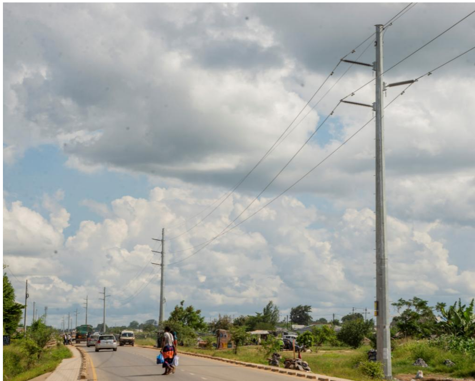
Construction of 132kV Single Circuit Transmission Line from Coventry – Waterworks, Coventry – Jimmy – Chawama for ZESCO in Lusaka
